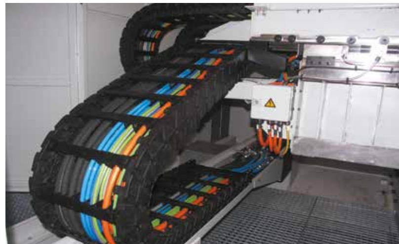
Chainflex® measuring system cable in a double-spindle horizontal machining centre.
