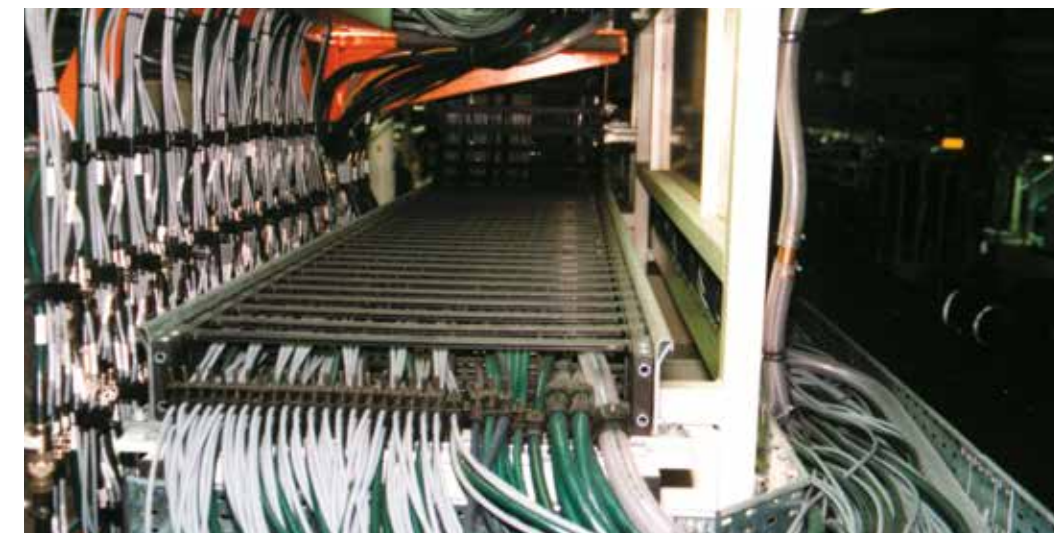
Chainflex® CF5 and CF6 control cables (green) as well as CF211 measuring system cables (gray) in a screwing station of a motor factory. E-Chain®: System E4/00 with chainfix clip strain relief devices
