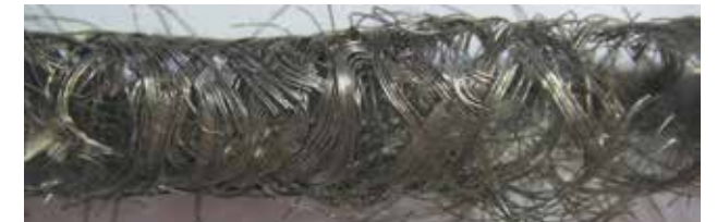
The detail inspection of the shield braid shows distinct damage on the shield wires.
