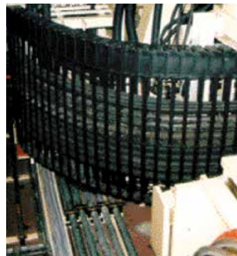
Hydraulics and electric cables are separated from one another in this example
