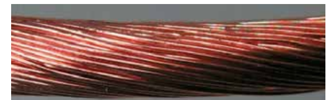
A close-up of the completely intact copper conductor. The inspection performed over the entire length shows that the conductor is still completely intact and does not have any individual wire breakages.
